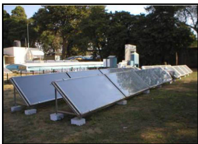
Figure.19 Solar air heating unit for drying system
